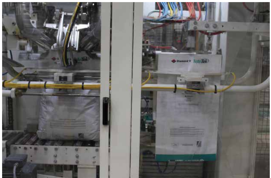
A new automated bagging system squares every bag it picks up before the bag gets hung and filled, ensuring a clean fill and consistent seal.
