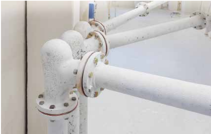
The plant has gone 16 years without an elbow failure after installing short radius deflection elbows on its pneumatic conveying lines.
