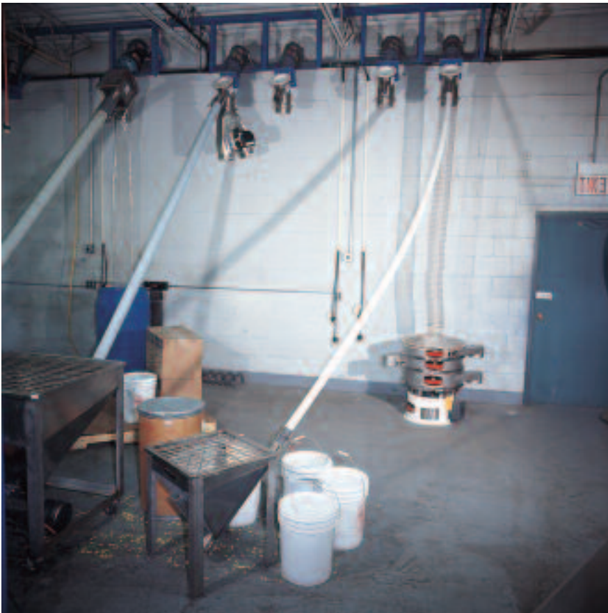
AFC plant officials duplicate the customer's plant conditions, such as feed rates and conveying angles, before conducting the tests.
