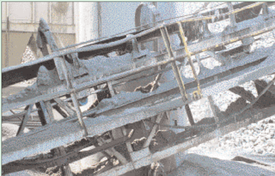
Preventing material buildup will help you avoid spillage like that piling up under this processed-sand belt conveyor.
